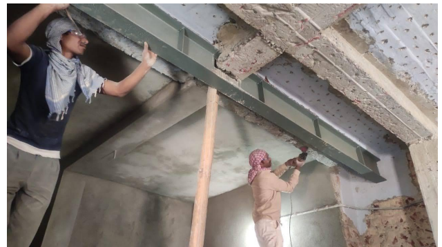
A new girder being placed in the ground floor classroom of Shanti Ashram.
